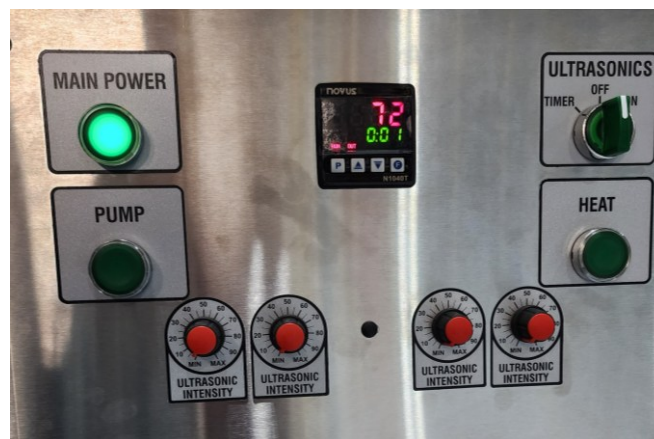
Figure 9: Ultrasonic Generators Turned Off
