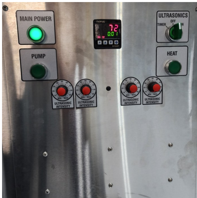
Figure 10: Generators Manual Control Off
