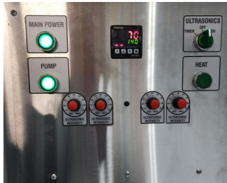
Figure 21 Pump Manual Control On
