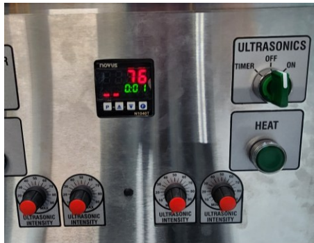
Figure 12: Generator Timer Off
