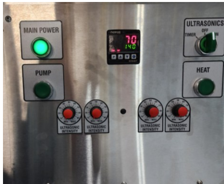
Figure 20 Pump Manual Control Off
