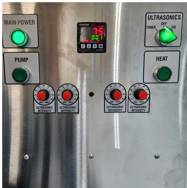
Figure 15: Generator Timer Running
