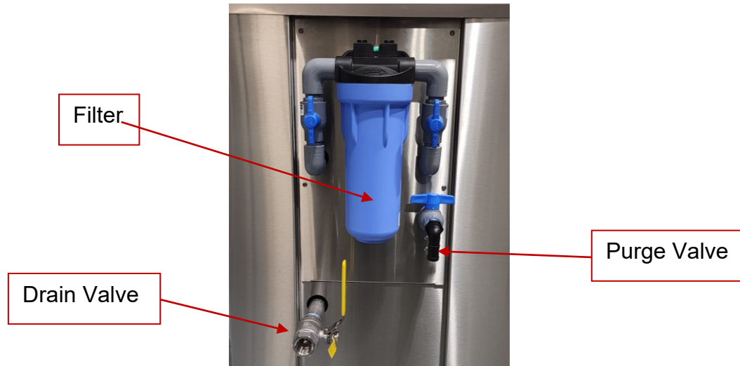
Figure 19: Filter, Purge Valve, and Drain Valve
